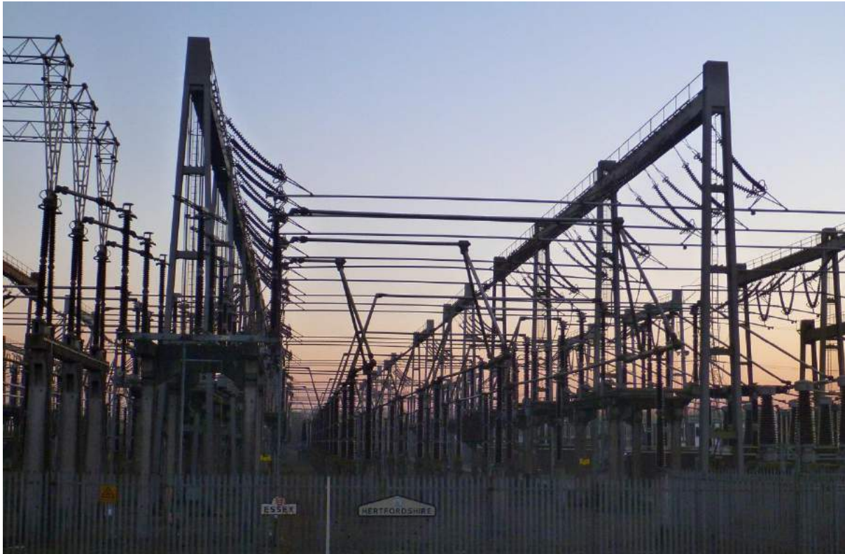
Fig 10: The Herts and Essex Electrical Transfer Station to the south of the Conservation Area has harmed its rural open setting.
